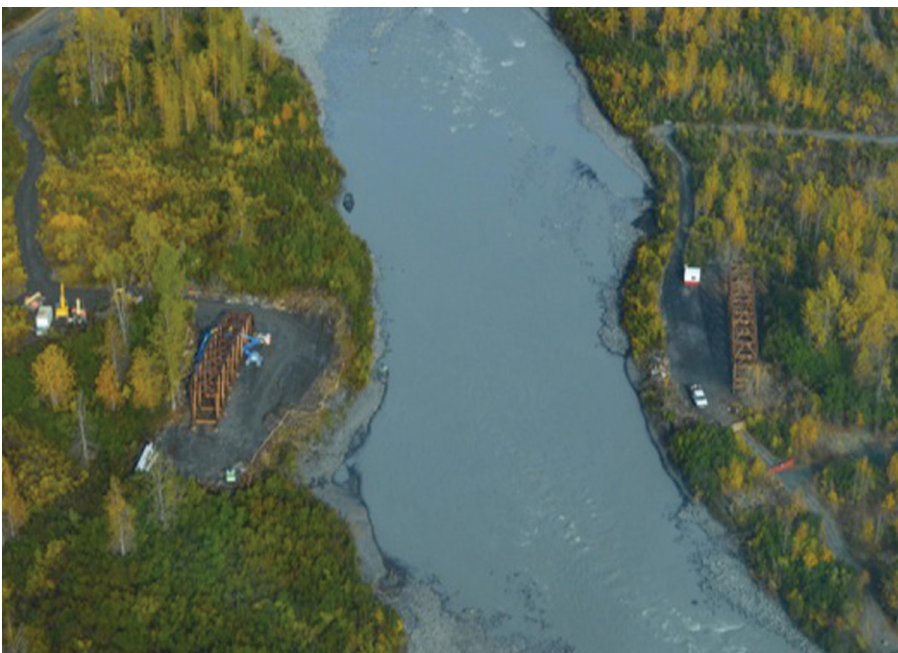
Because of the remote location and short weather windows, construction of the Placer River Trail Bridge spanned a period of three years. Photo courtesy of USDA Forest Service.
