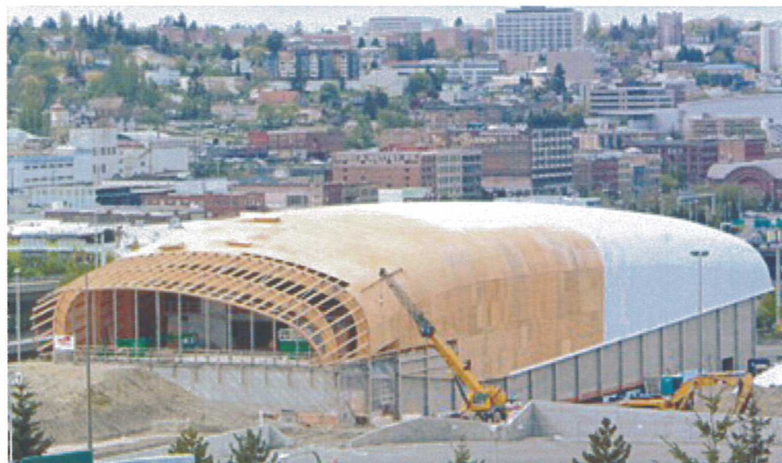
The curved roof, sheathed with fully sanded plywood, is streamlined like the aerodynamic surfaces of an automobile.
