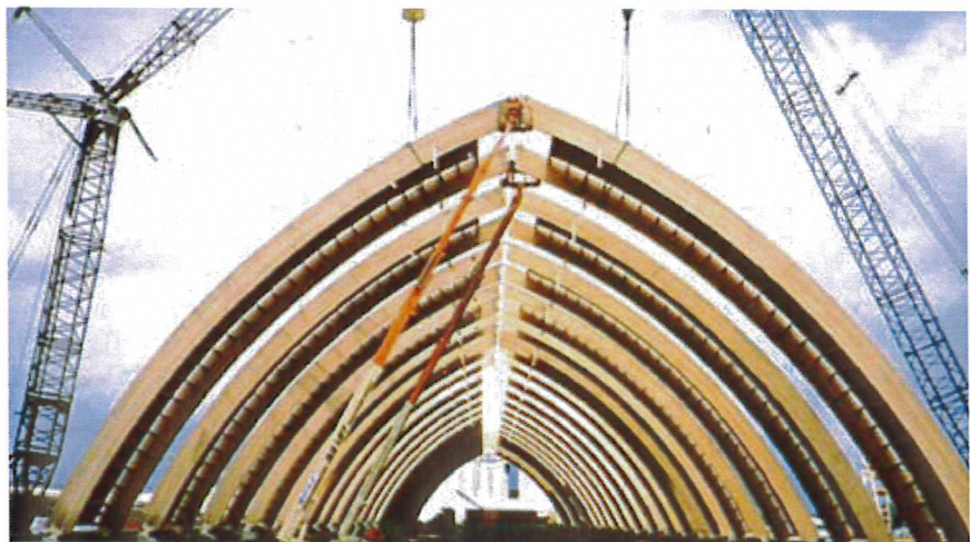
The 236,000 square foot potash storage building in Portland, Oregon features APA EWS glulam arches in its design.
