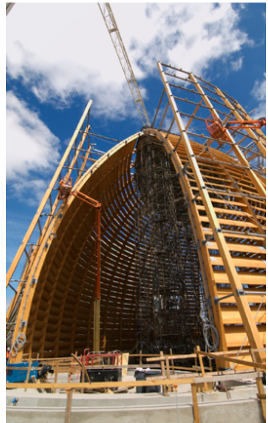
Given the asymmetry of structure and the curvature of the interior and exterior walls, very few connections were the same. As a result, AutoCAD 3D was utilized to model 220 unique connections. © John Blaustein 2008.
