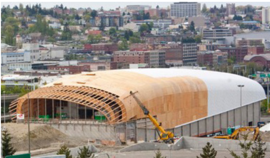
The curved roof, sheathed with fully sanded plywood, is streamlined like the aerodynamic surfaces of an automobile.
