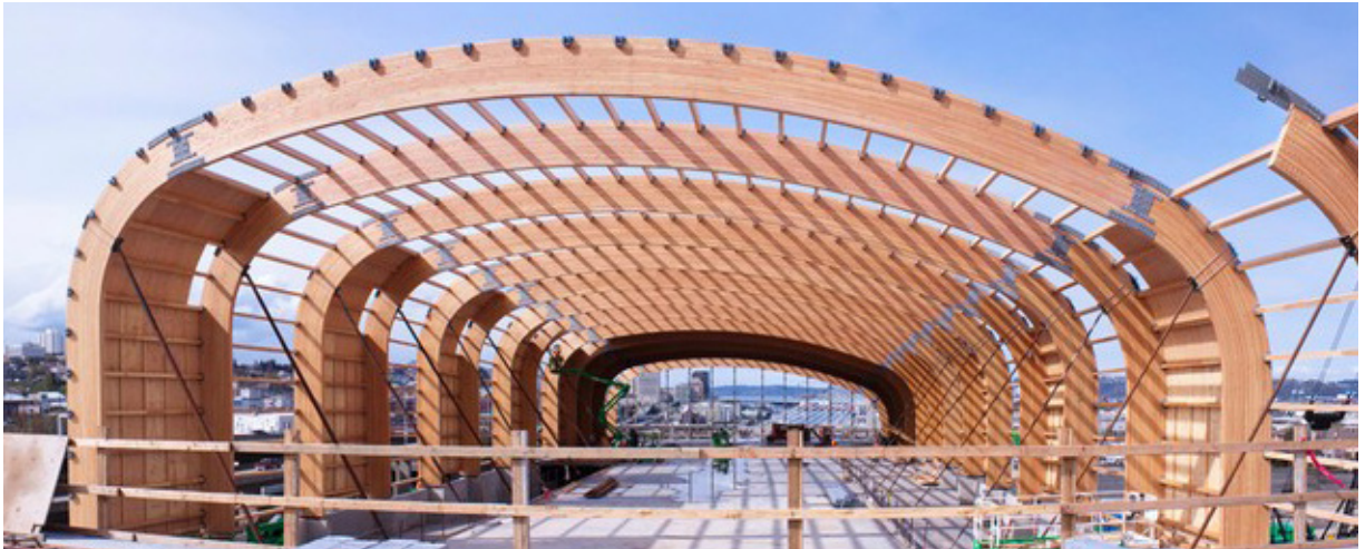
Glulam beams are erected to create the arched curve profile of the LeMay Museum roof, shown during construction in Spring 2011.
